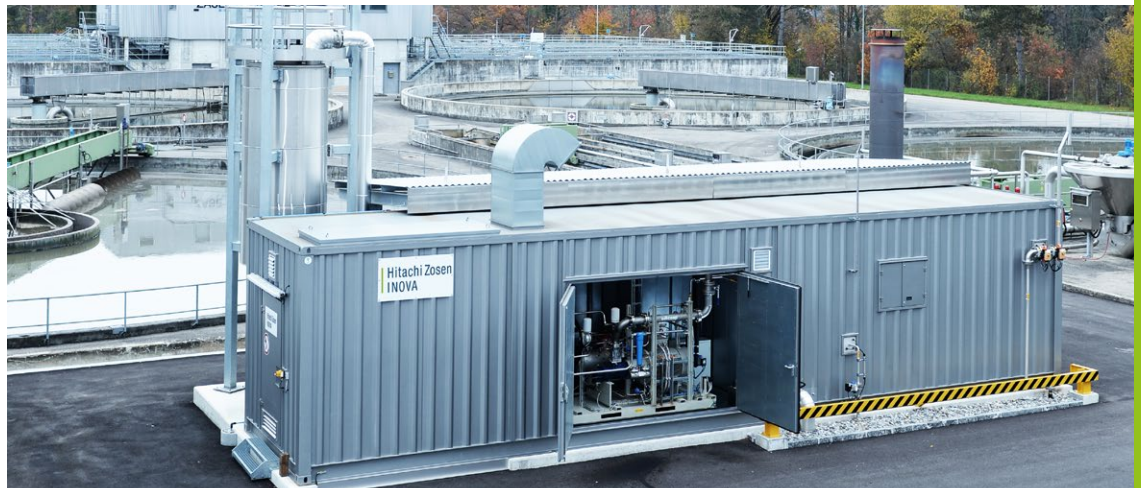
Using membrane technology to treat sewage gas in Zuchwil, Switzerland
