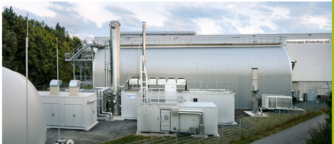
Biogas treatment in Winterthur, Switzerland, using Kompogas® dry fermentation with amine scrubbing
